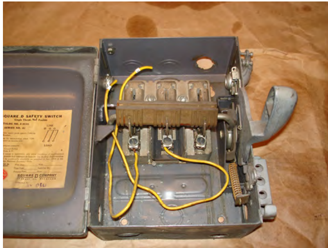
Figure 97: Safety switch before refurbishing.
